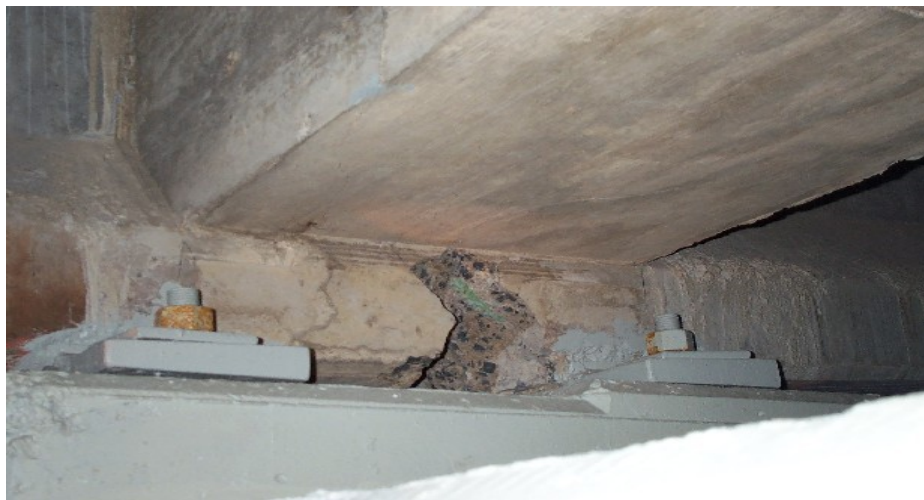
Figure C31- Crack and spall at diaphragm over pier support
