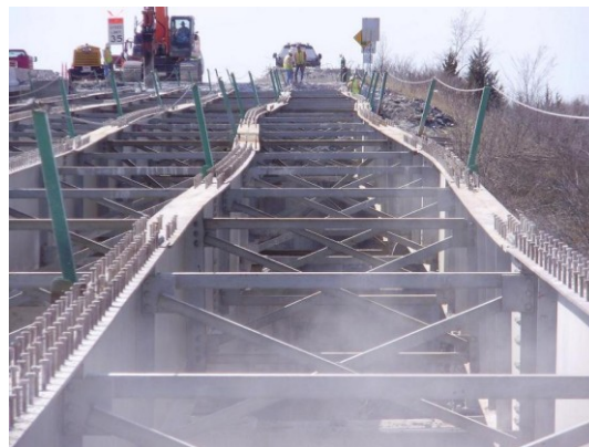
Figure C62- Improper deck removal
