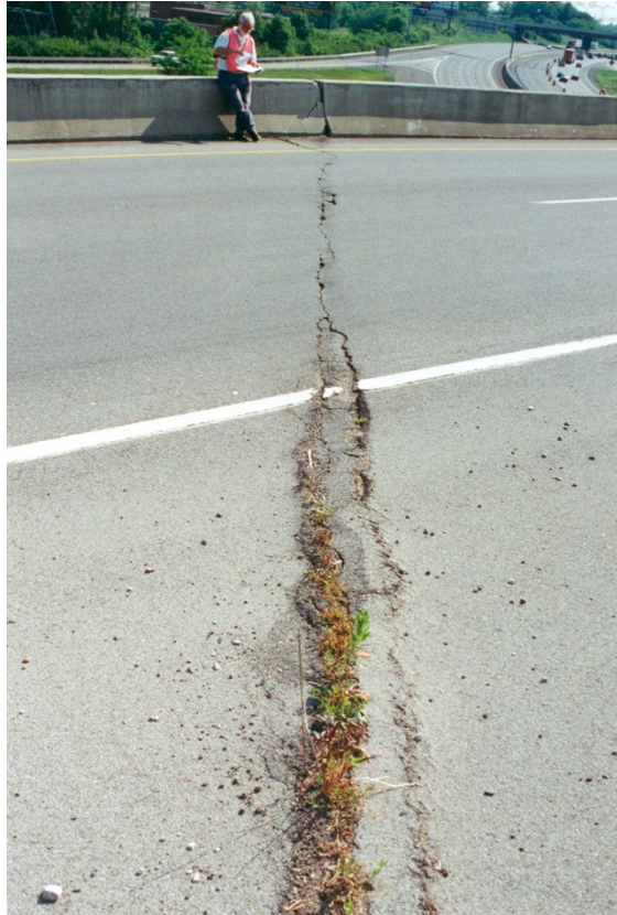
Figure C19- Asphalt overlay distress (west end) (Tabatabai, Oesterle and Lawson, 2005).
