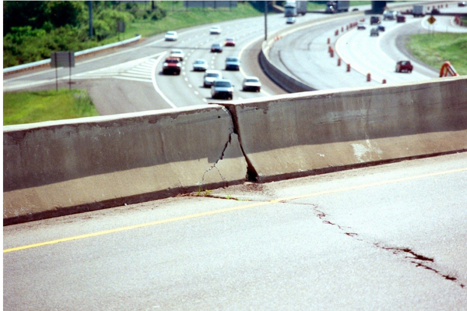
Figure C20- Barrier distress at west abutment (Tabatabai, Oesterle and Lawson, 2005).
