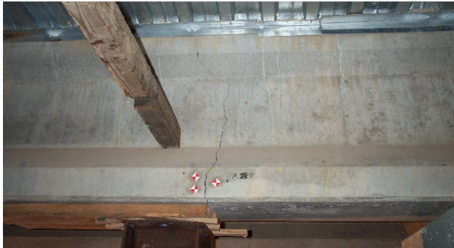
Figure C30- Cracks near girder supports
