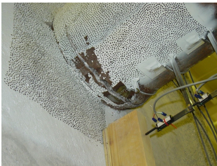
Figure 4-27- Crack completely opened at load stage 3-19 ( \pm 4.75 in)
