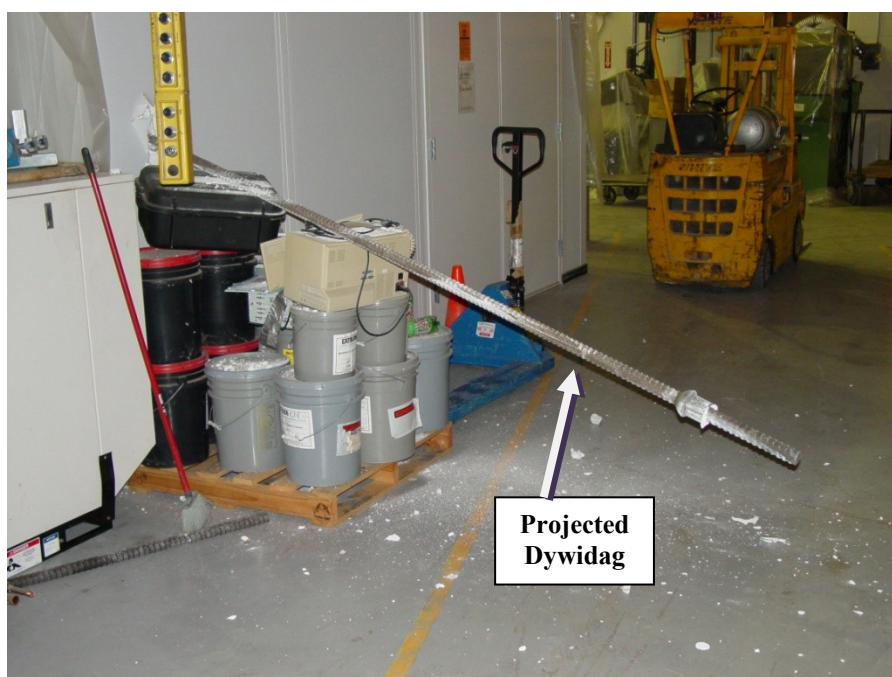
Figure 4-35- Failure of the dywidag
